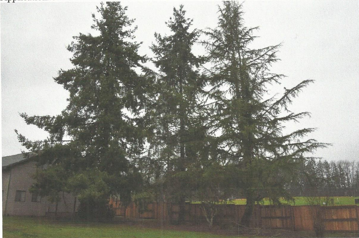
Trees on the east side. Tip dieback can be seen in the trees.
