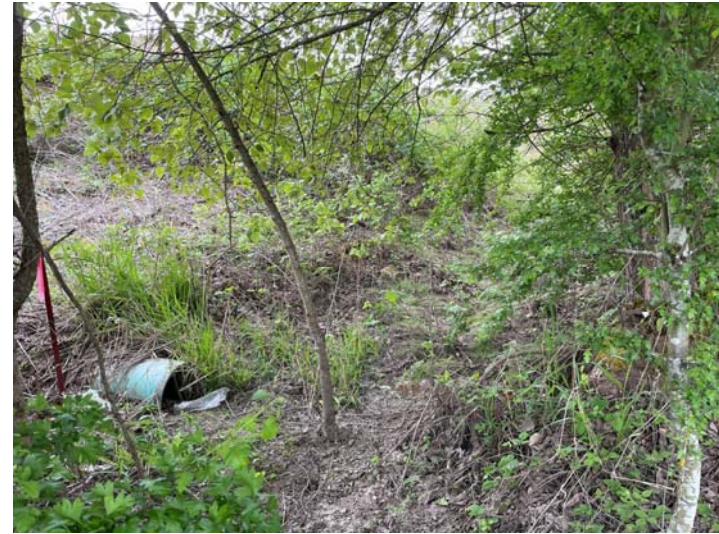
Photo F. View east of Plot 9 and existing culvert showing no evidence of defined bed and bank, OHWM, or signs of recent surface water flow.
