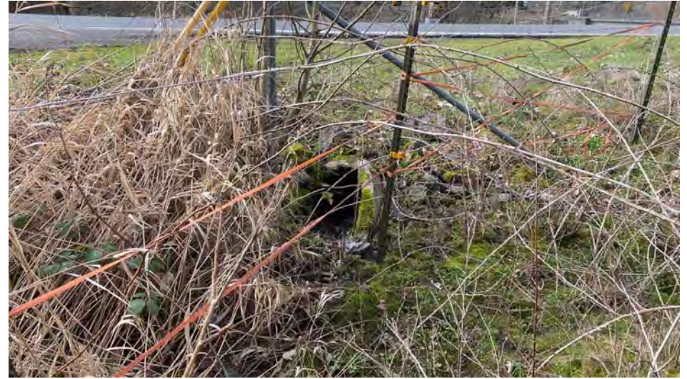
Photo J. View of culvert under SW Tonquin Road within Wetland A.
